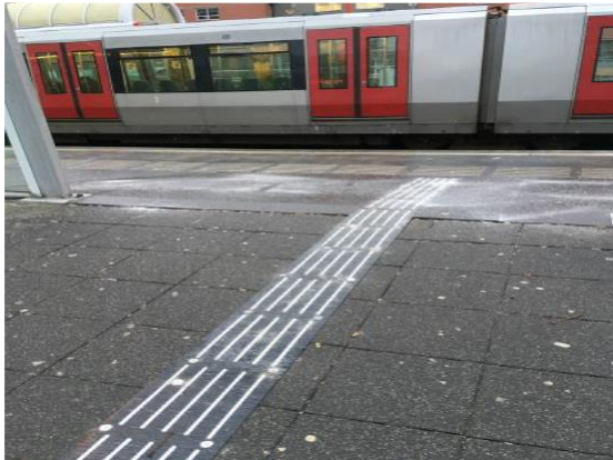
Plug/ schroef-en-ring verbinding in betontegels.
